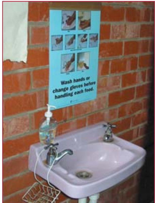
Photo 11. Hand washing facilities should be provided with instruction to employees
