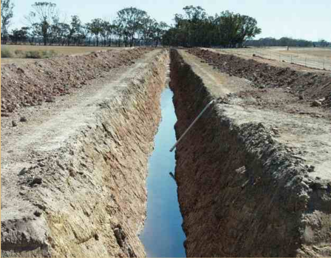
A double leaved deep drain with surface water inlet pipe. Surface water can be drained from outside the spoil bank by piped inlets that extend through the bank at ground level and discharge into the drain.
